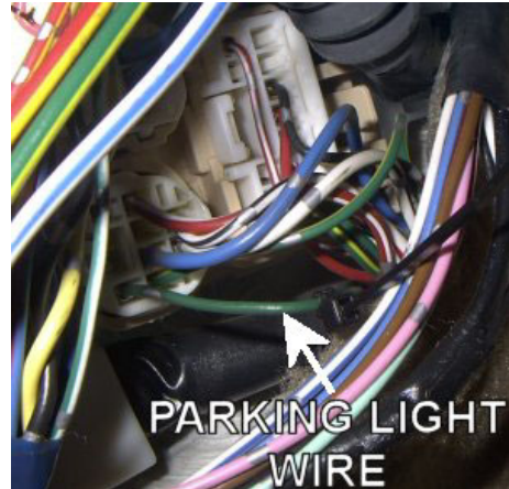
Pictured is the location of the parking light wire in the driver's kick panel of a 1999 Toyota Avalon.
